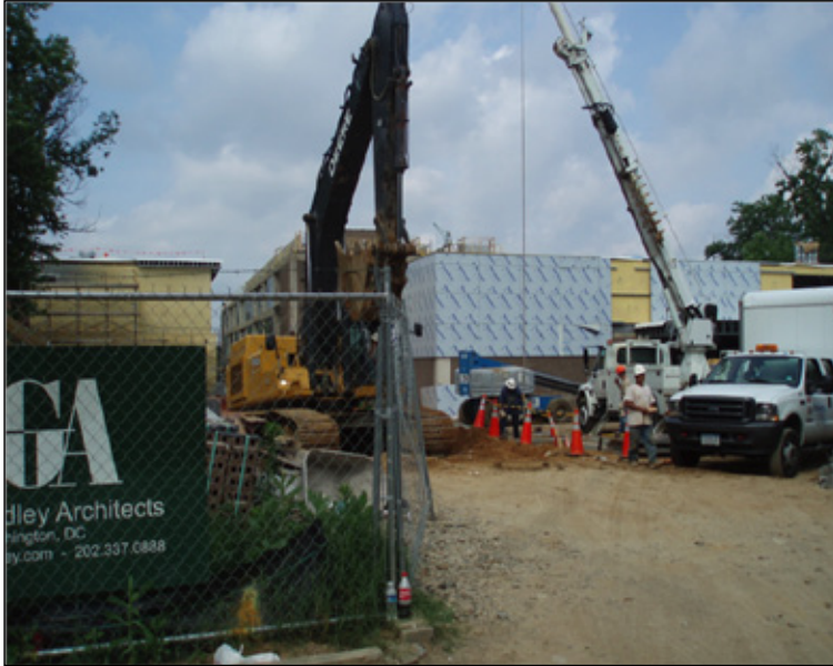
Addition on a 1960s public school, being modernized in 2009 (Source: 21st Century School Fund, 2009).
